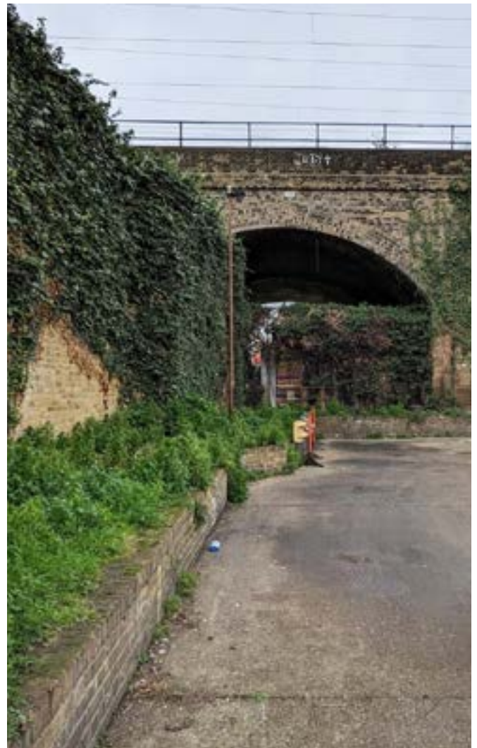
Fig 6: photograph from inside the bus garage looking east along the northern boundary into a railway arch
