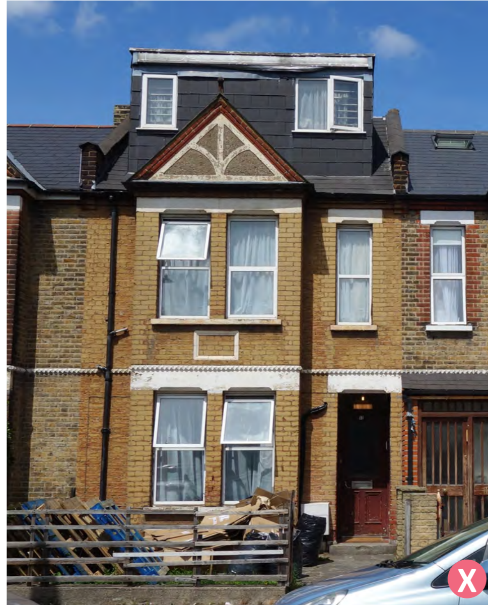
Fig.21: The additional level is out of proportion with the host house
