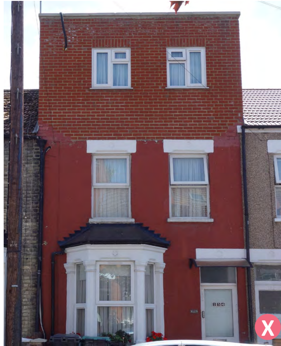
Fig.35: The roof extension windows are not in keeping with the existing window shape, size and alignment.
