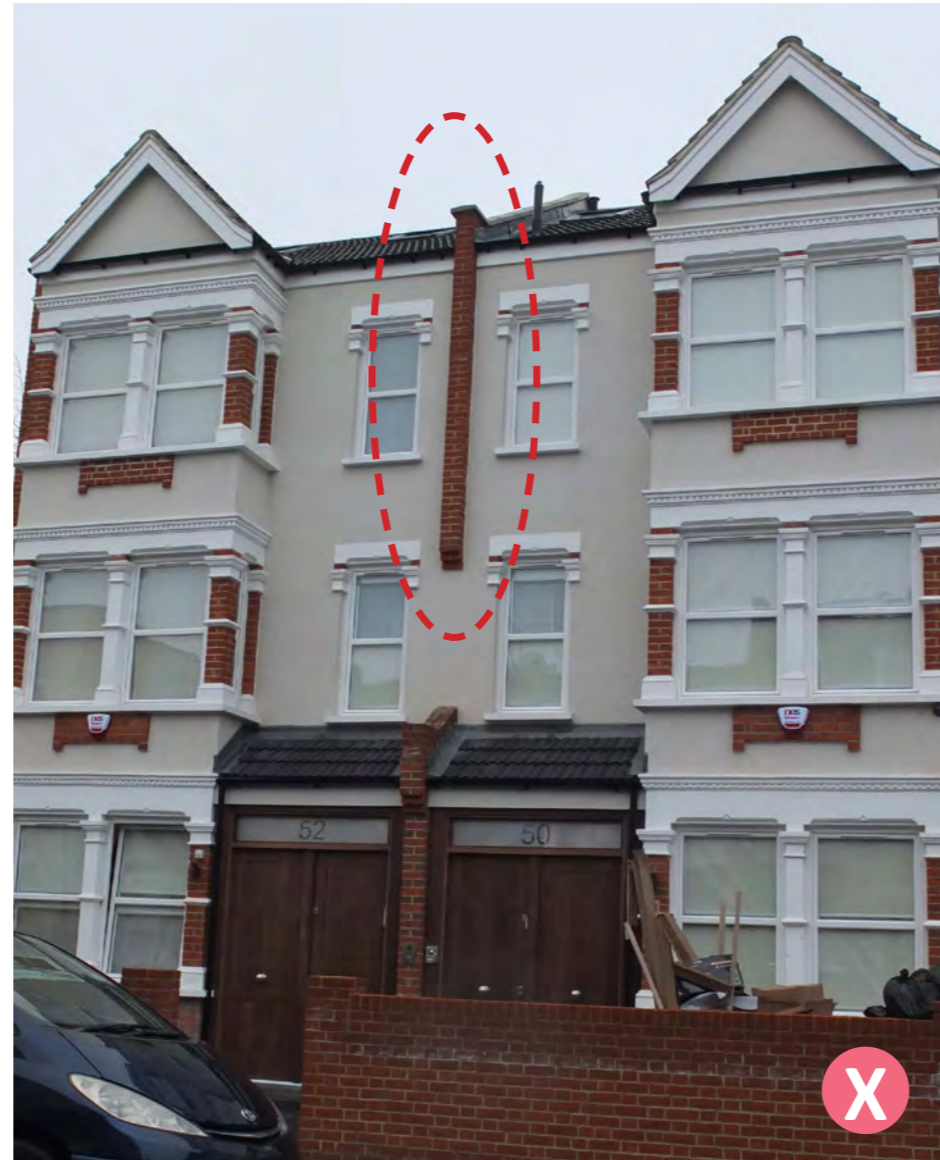
Fig.33: An unacceptable example of a party wall has been corbelled out, not in keeping with the original architectural detailing
