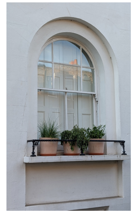
Arched window to ground level, metalwork to base of window.
