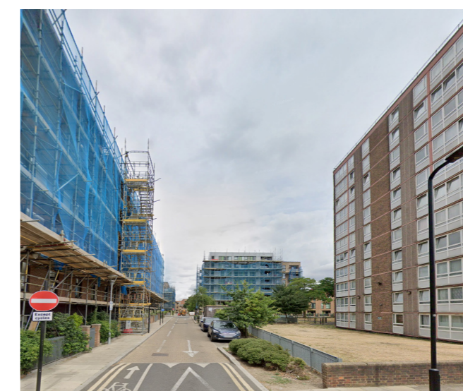
Existing example of a 22m gap between 11-storey Bryant Court and a 6-storey development located 200m from Fellows Court
